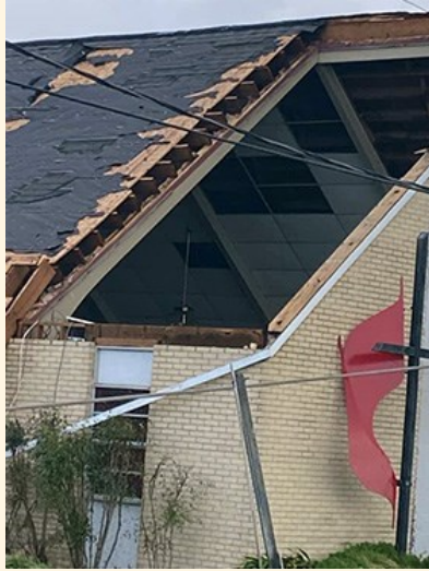
The sanctuary at Golden Meadow United Methodist Church in Galliano, La., stands open to the sky after Hurricane Ida tore off part of the roof. Photo courtesy of the Louisiana Conference.
